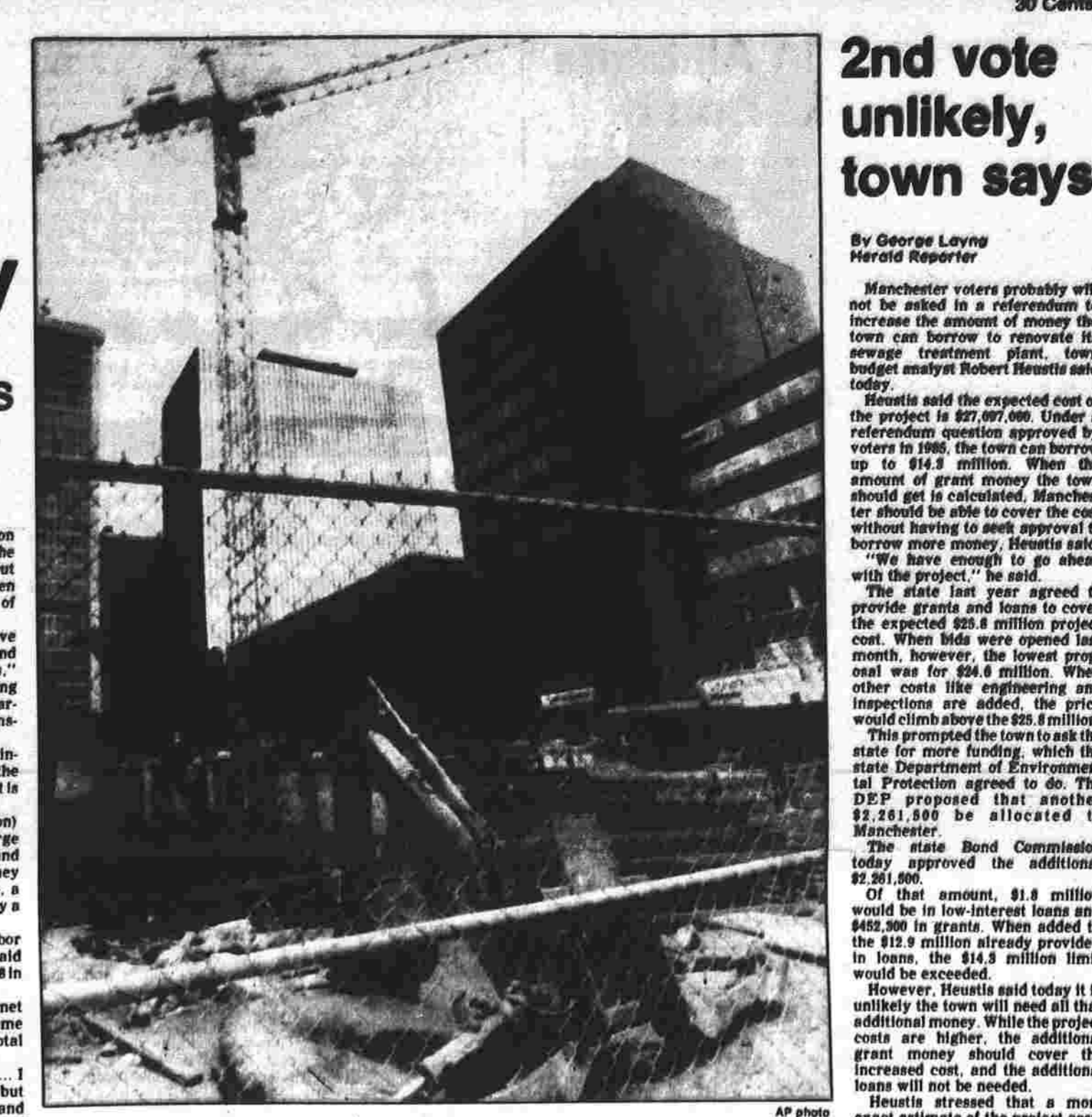
The site of a new bank in Hartford sits statewide strike has shut down or idled as a result of a strike by members of the Union of Operating Engineers. The AP photo
